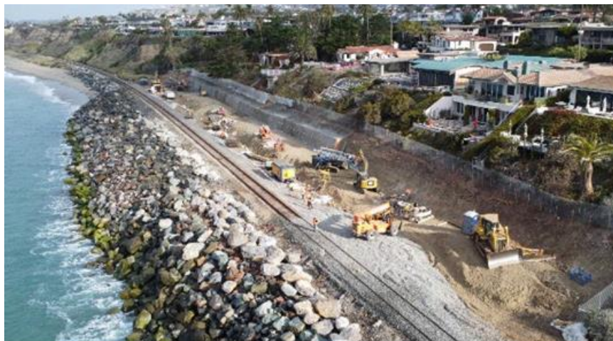
3. Impacts of erosion of bluffs along the LOSSAN Rail Corridor
